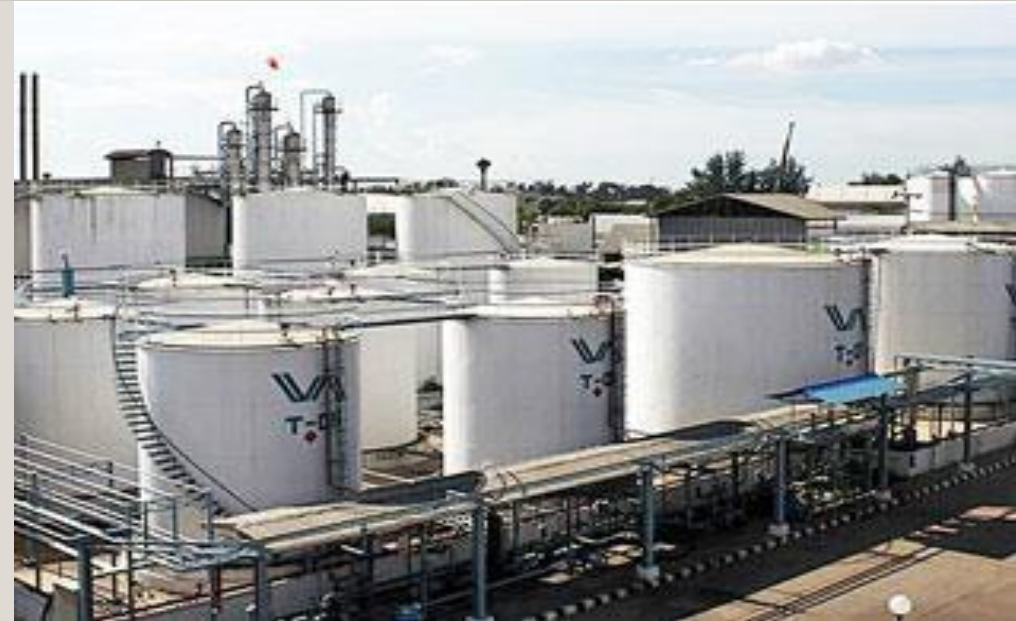
Verasuwan oil & gas facilities
